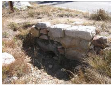
Partially blocked culvert.
