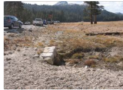
Culvert set too low in meadow.
