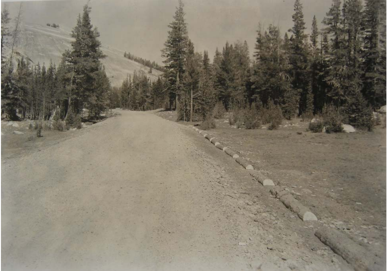
Figure 1-4. The realigned Tioga Pass Road through Tuolumne Meadows, under construction in 1935. Note small lodgepole pines near the road, but not significant numbers of seedlings in bare areas along the shoulder. Negative number ECW1311. Source: Yosemite Research Library.
