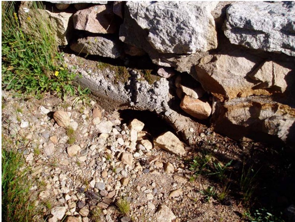
Figure 2-17. Example of culvert filled in with sediment, which obstructs water flow. Filled culverts are more common on the east end on the meadow.
