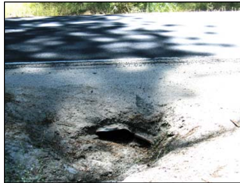
Dysfunctional culvert at El Capitan Straight
