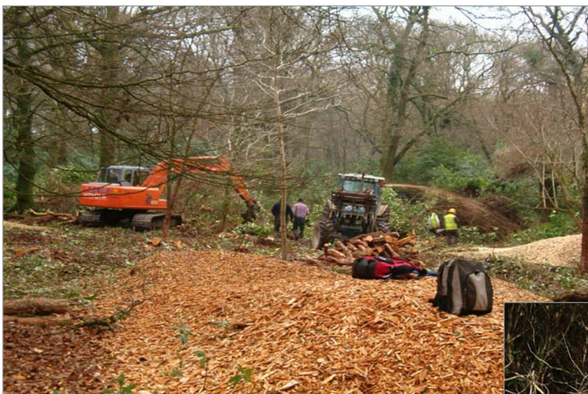
Stumps can be extracted with a bucket, mounted on a track machine.
