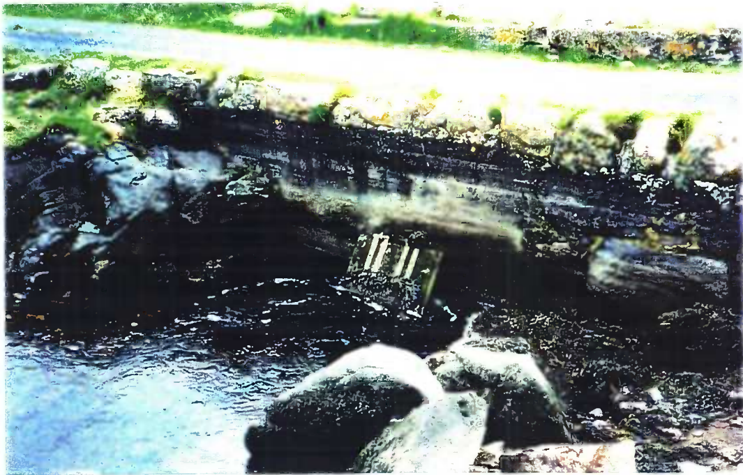
Plate 4.12.1 View of the sluice at the northern end of the lough (Sta. 1) Maghery Lough, Co. Donegal, 1998.
