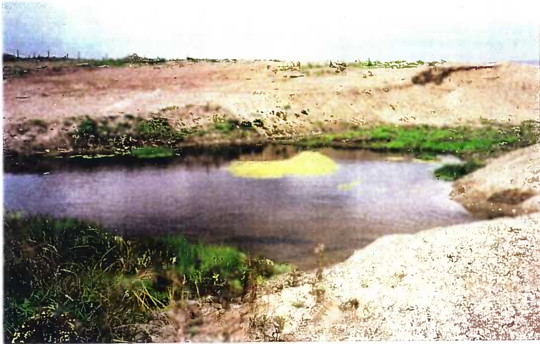
Plate 4.1.5 View of one of the gravel pits being excavated (Sta. 4), Ballyteige drainage channels, Co. Wexford. 1998.
