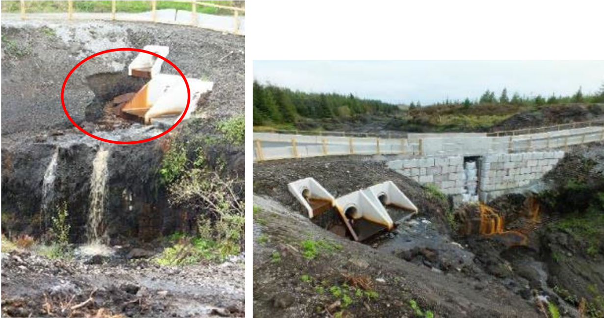
Figure 8-3 Eroding Banks at Culverts of Dawn of Hope Bridge
