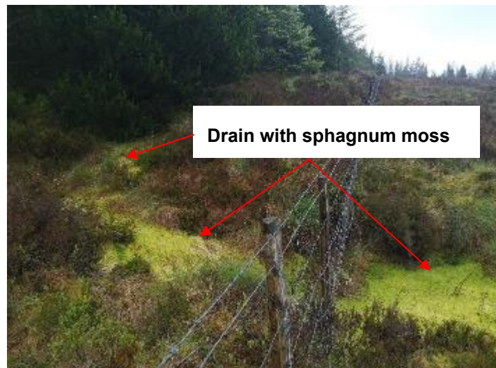
Figure 5-1 Perimeter drain revegetated with sphagnum moss on the edge of the forestry at Shass Mountain
