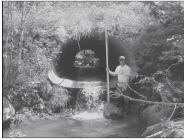
Barriers, such as culverts, can prevent wildlife from moving up and down Vermont's streams and rivers.
