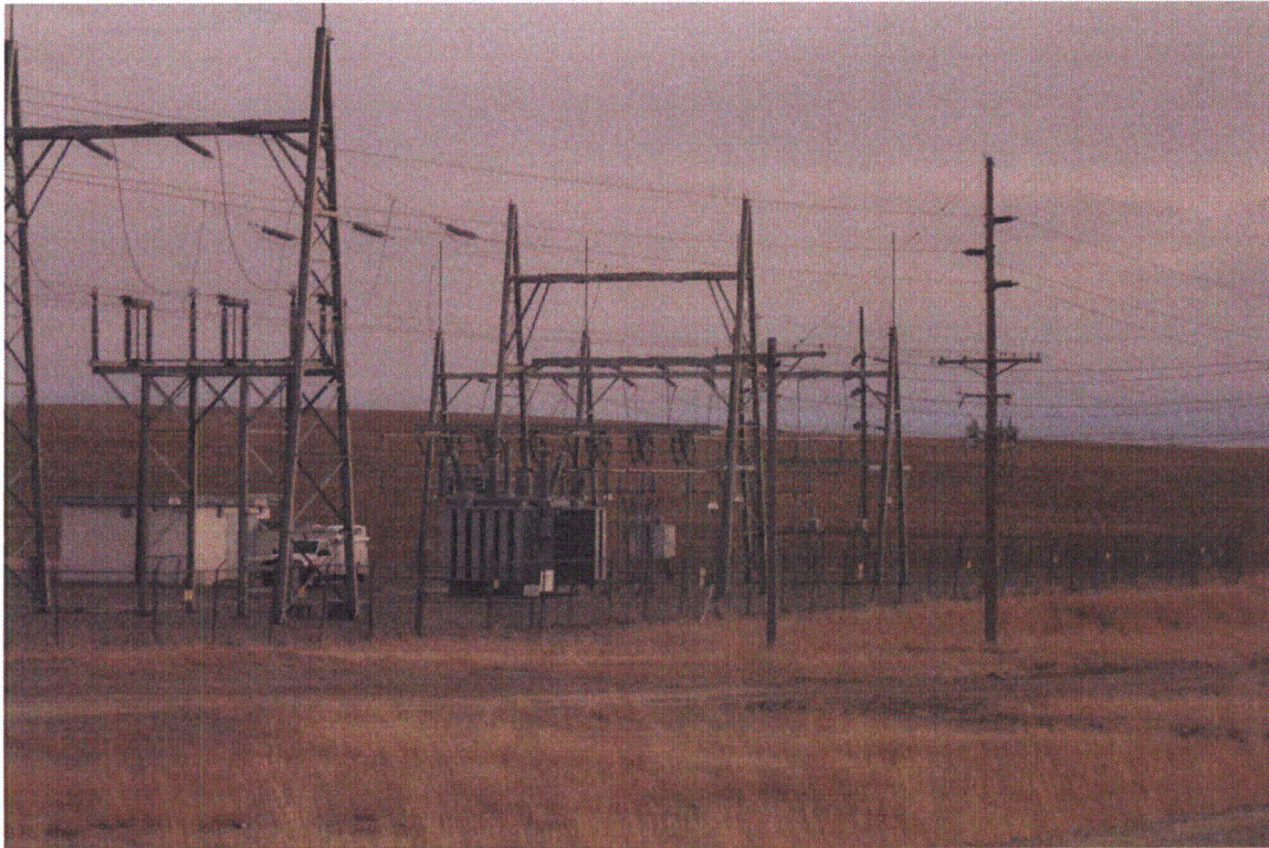
Figure H-5b. Bonneville Substation, facing northeast.
