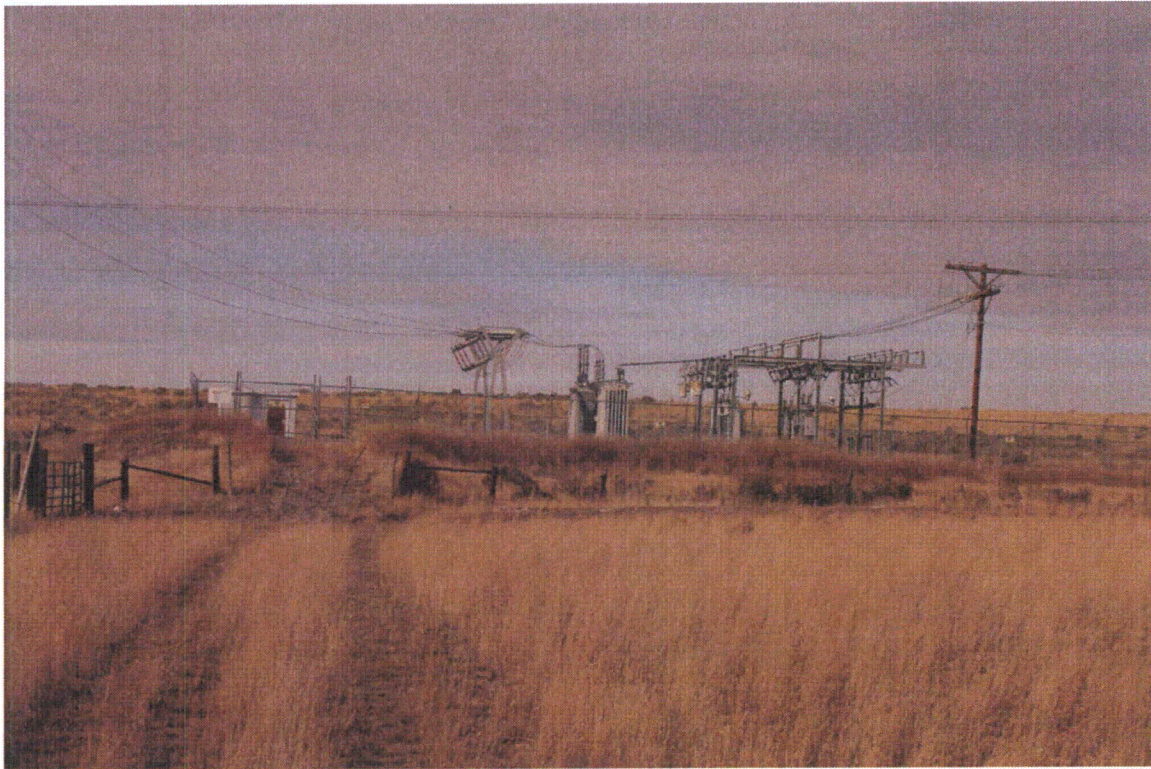
Figure H-5c. Kettle Substation, facing west.
