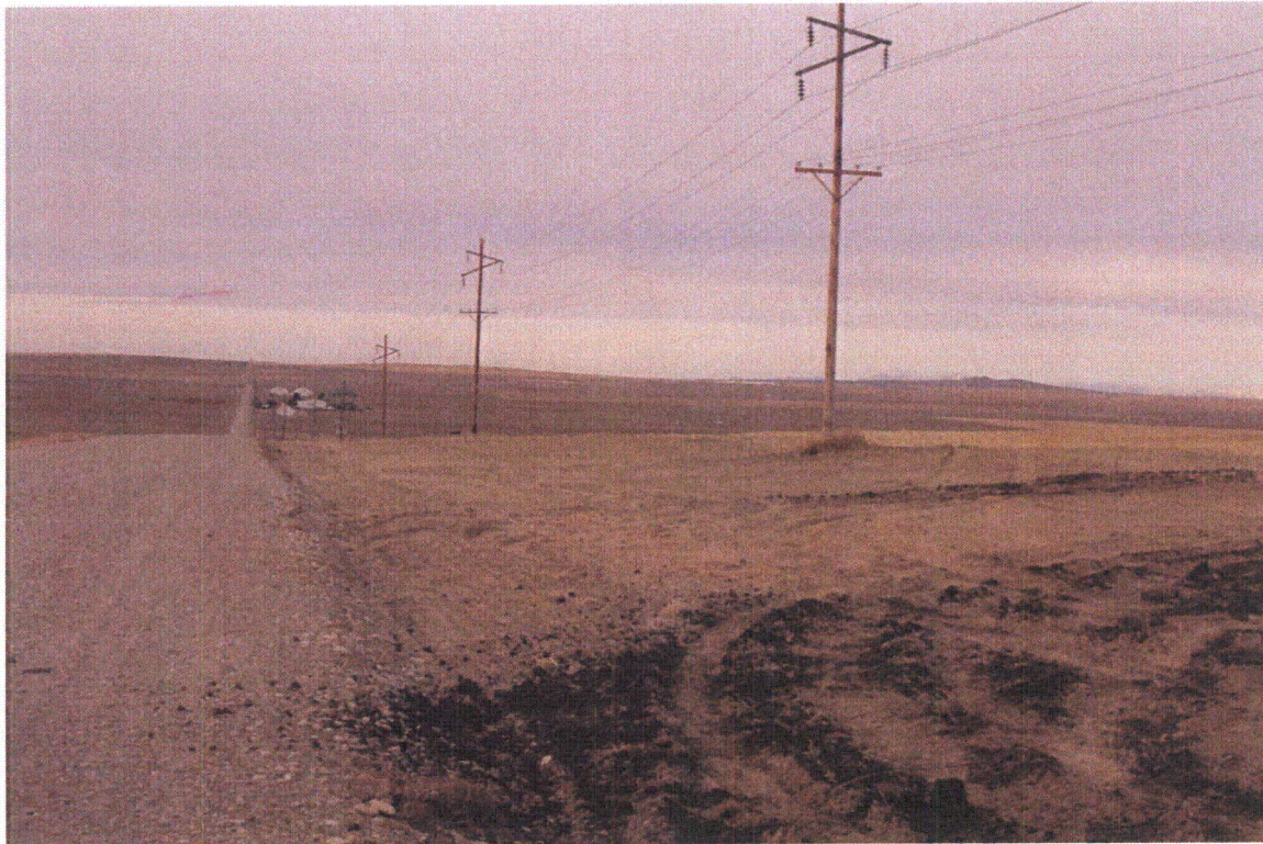
Figure H-5a. Existing 69-kV transmission line along county road West 65 North Street, from Bonneville Substation to the Kettle Substation, facing west. Note agricultural fields that extend to the road edge.
