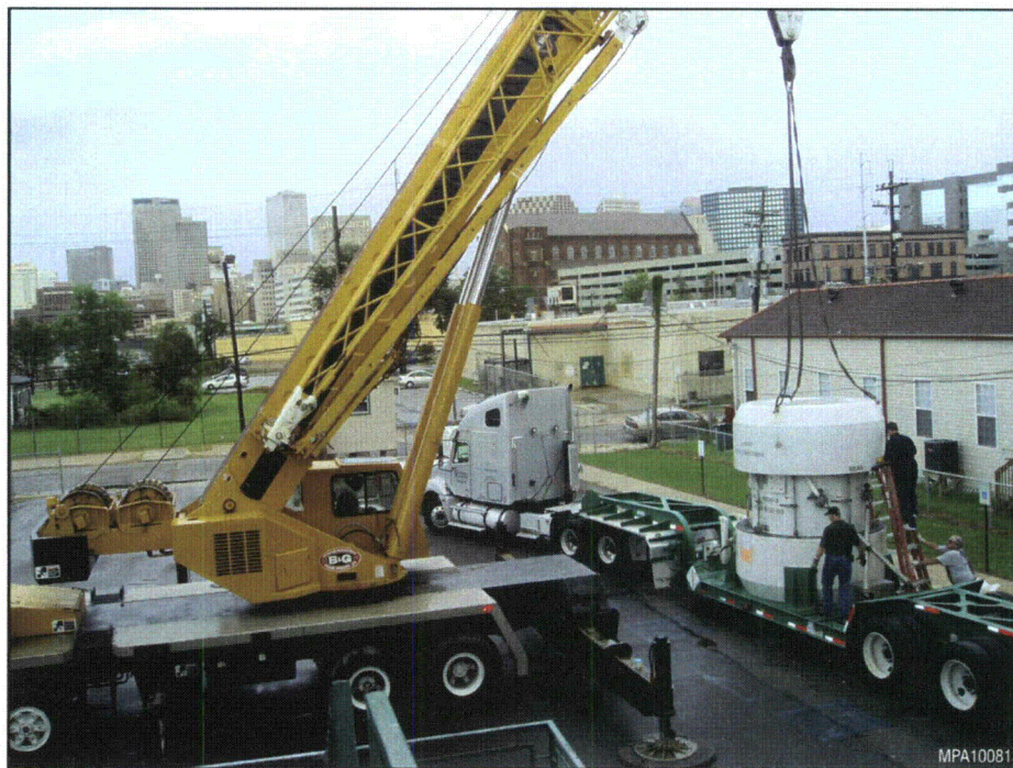
25 26 FIGURE 5.2.9-1 Transport of Radioactive Waste Containers 27
