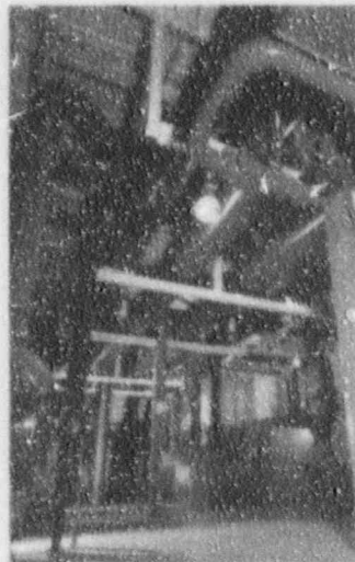
Three million 100-ton gallons of water will circulate each day and chilled water in the new Allegheny Development Corporation's central energy facility.
