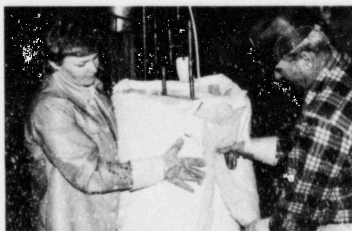
WATER HEATER INSULATION JACKET PROGRAM — Ginny Joles, Consumer Services and Information Representative, and Adam Albert, Caribou District Leadworker install a free water heater insulation jacket in a Caribou home.
