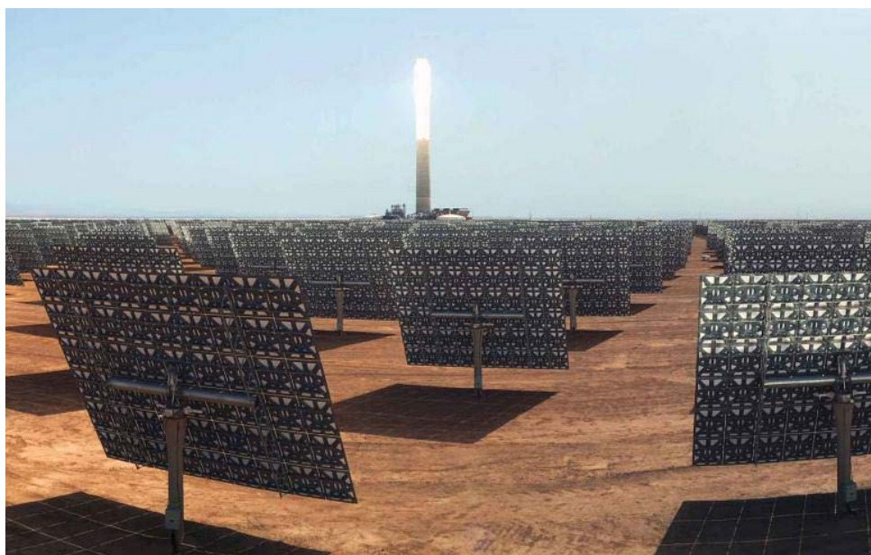
Figure 16. SENER's HE54 heliostats at Morocco's Noor III facility (operational since 2018)
