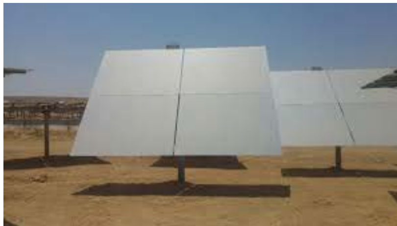
Figure 20. Wireless BrightSource heliostat at Ashlim with top-mounted PV panel
