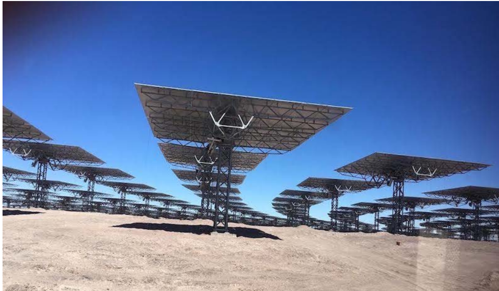
Figure 18. Abengoa trussed heliostat at Atacama I
