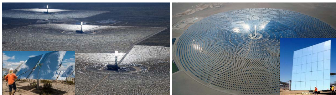
Figure 1. Heliostat size varies widely at deployed U.S.-based utility-scale power tower plants—ranging, for example, from 14 m 2 at Ivanpah (left), to over 100 m 2 at Crescent Dunes (right). HelioCon will advance an established heliostat design and manufacturing approach within the United States.
