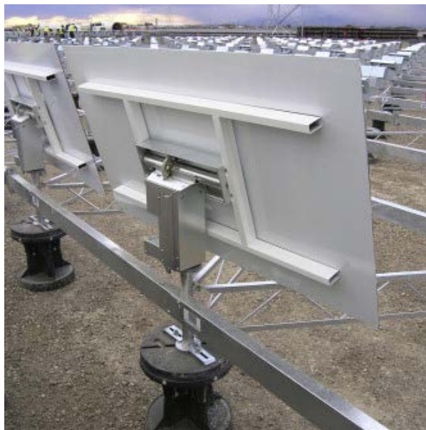
Figure 17. eSolar trussed and ballasted heliostat
