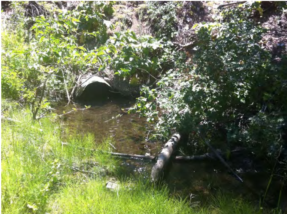
Photo 10: View of actively flowing creek channel mapped as other waters at the culvert opening under Old U.S. Route 50. June 28, 2012.
