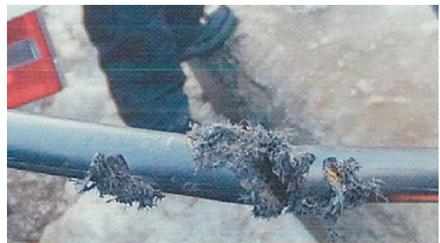
Fig. 2. Damaged optical cable with open cut.
