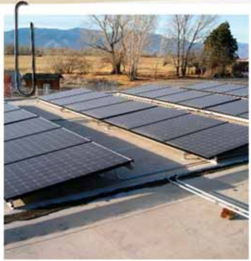
The Washoe Tribe received a rebate check for $33,185 for installing solar panels on their office building.
