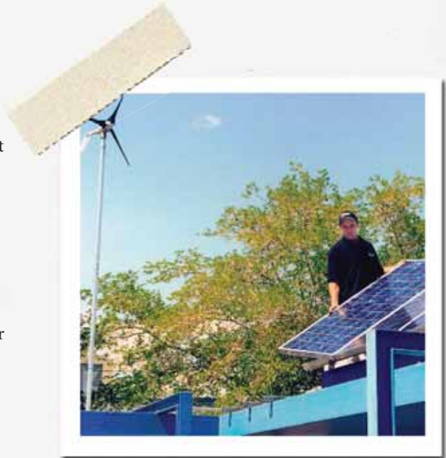
Solar installation at Hyde Park Middle School in Las Vegas.
