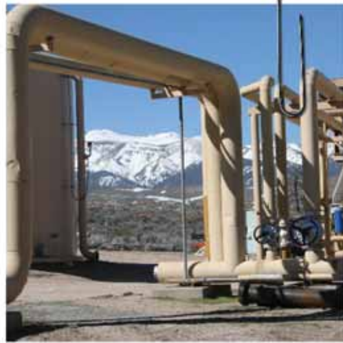
Ormat geothermal facility, Steamboat Nevada.
