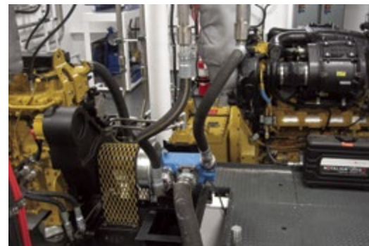
M/V Manu'atele's massive GenSet - a pair of 99 kW Caterpillar C4.4s.
