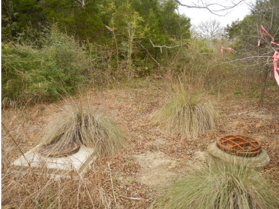
Photograph 35: Utility infrastructure within the Bee Cave detention pond; facing west.
