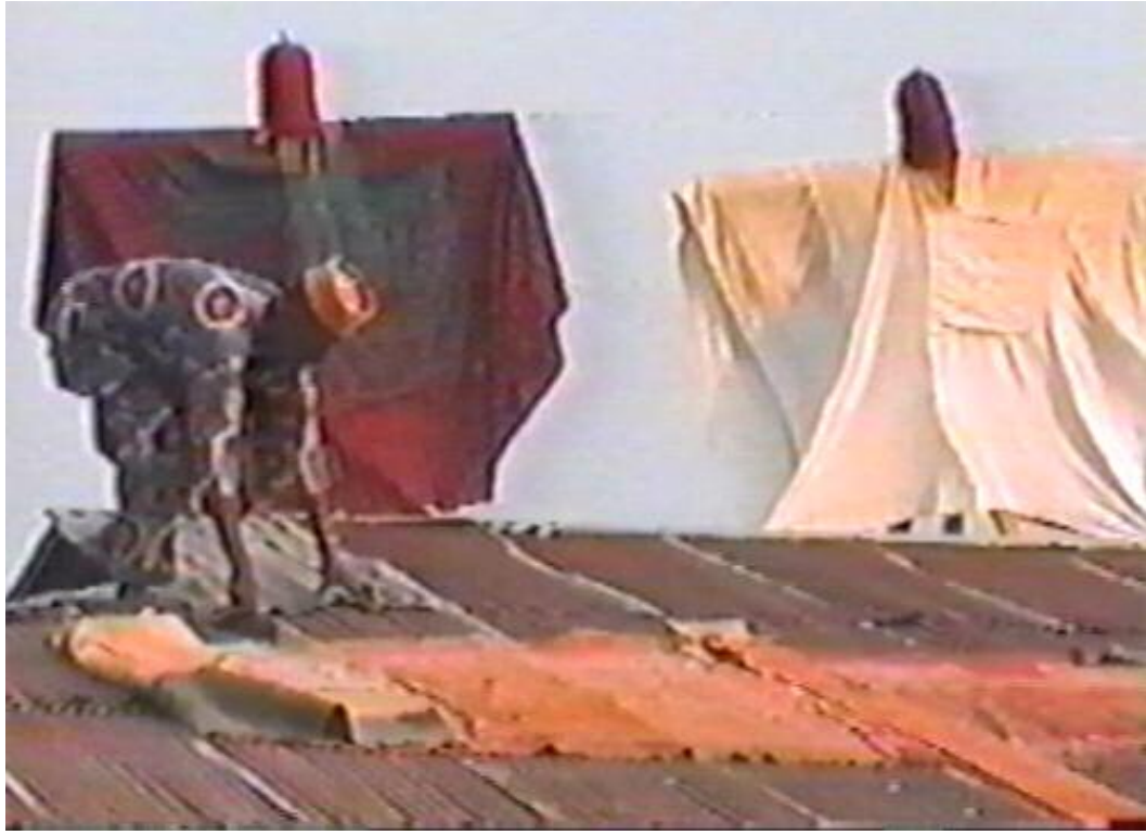
Figure 4.3: A carpenter detaching the Ogalata items on the late Chief Olugbami's house roof. Ekinrin-Adde, December 2000. Still photograph adapted from video documentation; courtesy of Chief S.A. Olugbami.
