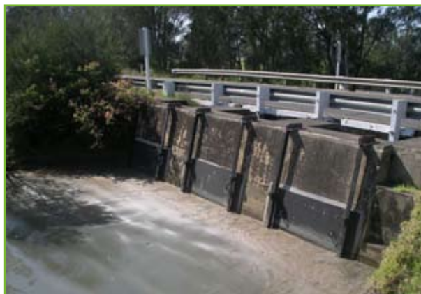
Floodgates on Crookhaven River NSW, source: NSW DPI (T Townsend)
