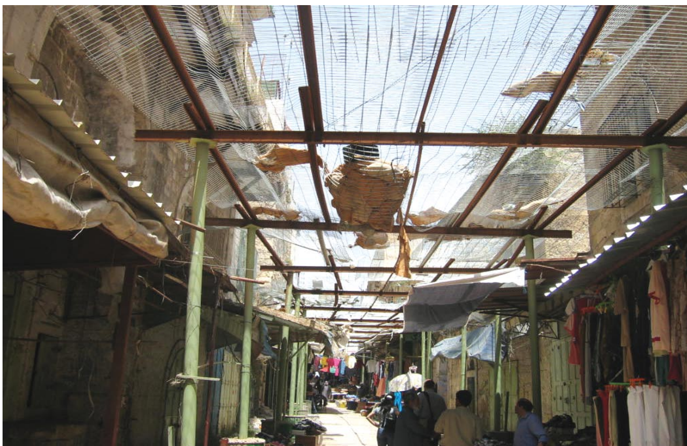
Settlers occupy the second storey of these buildings and throw garbage and human excrement onto the street lined with Palestinian shops and houses below. Palestinians have been forced to put up wire mesh to stop solid objects hitting people passing. Photo by OCHA / Steve Sabella, 2005.
