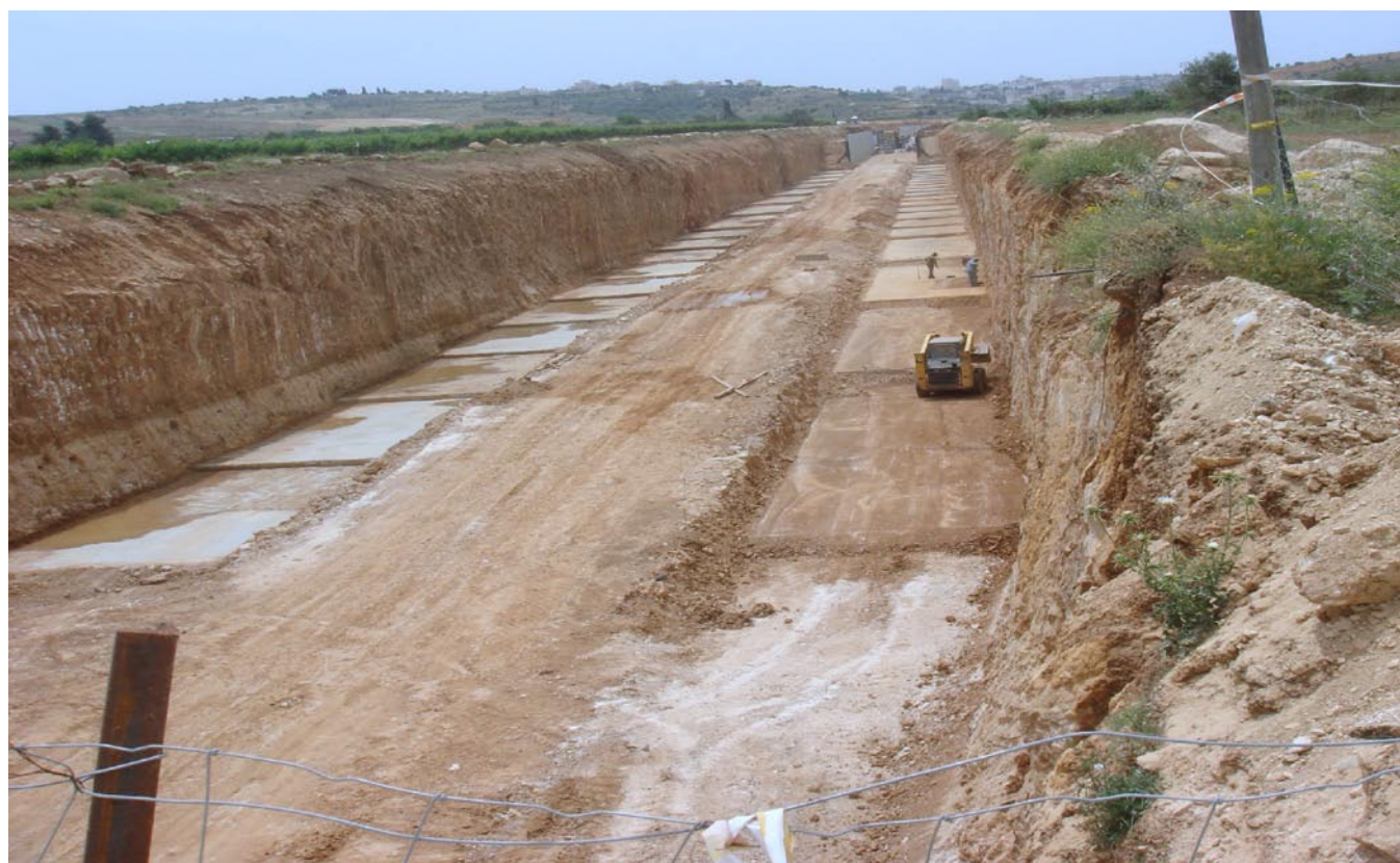
Palestinians wishing to leave the Bir Nabala and Biddu enclaves to travel to Ramallah will need to use a sunken road (under construction) to pass under Road 437, a road reserved for Israeli use. Photo by OCHA, 2007.
