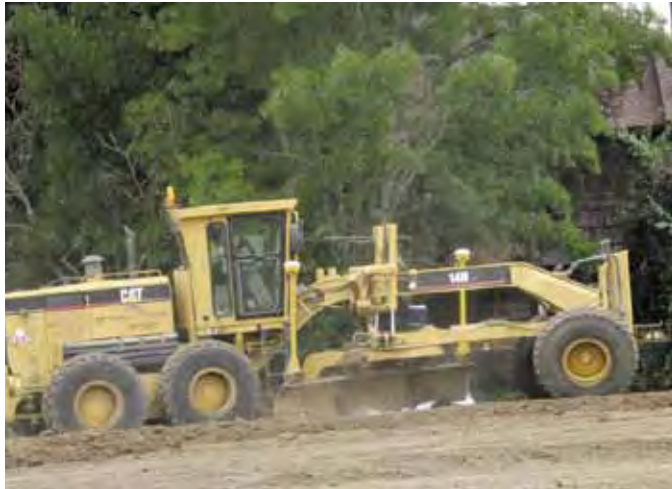
Blade Operator Kevin Uffelman clears the area surrounding the much-anticipated Brookfield Homes subdivision in Rohnert Park.
