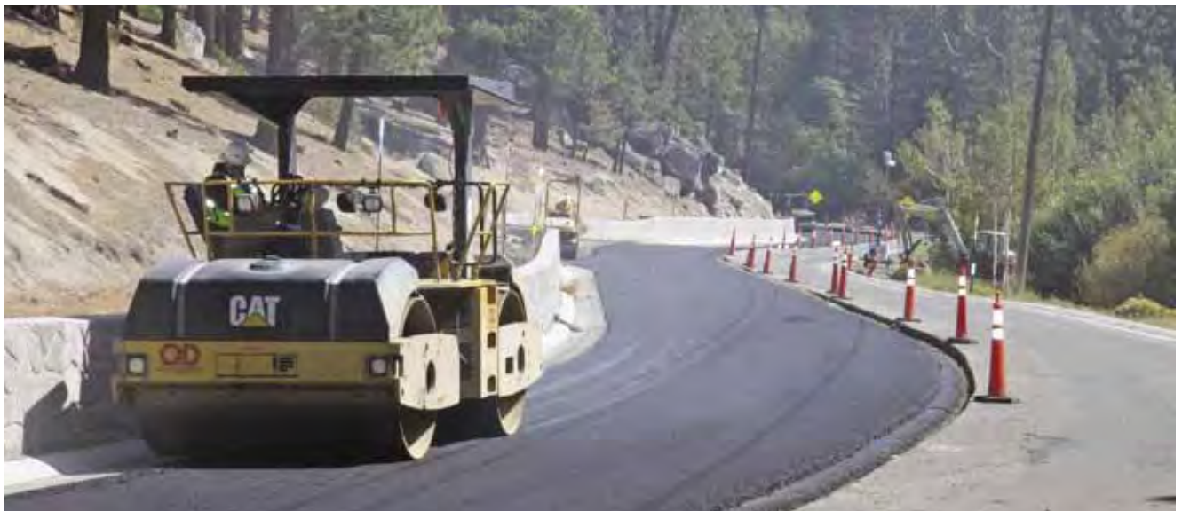
From left: Roller operators Cliff Birdsall, Neo Velazquez and Vince Greco stay in sync as they follow the paver down the highway.
