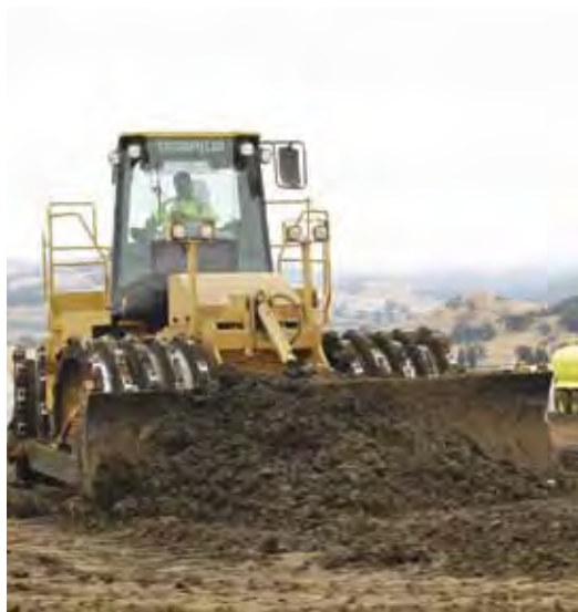
Compactor Operator Etuate Faiva prepares the ground for nearly 1,700 homes in Rohnert Park.
