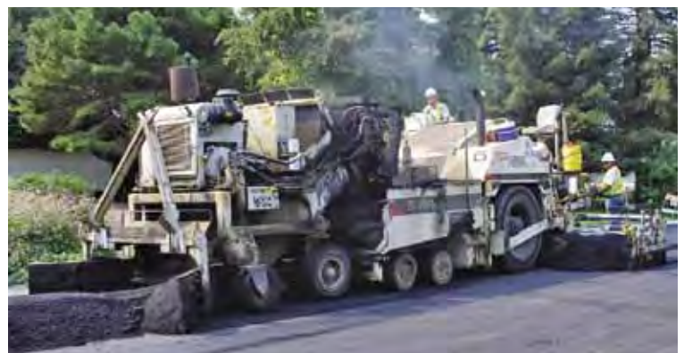
Lyle Swartz works on a paving job in Yuba City for Teichert.
