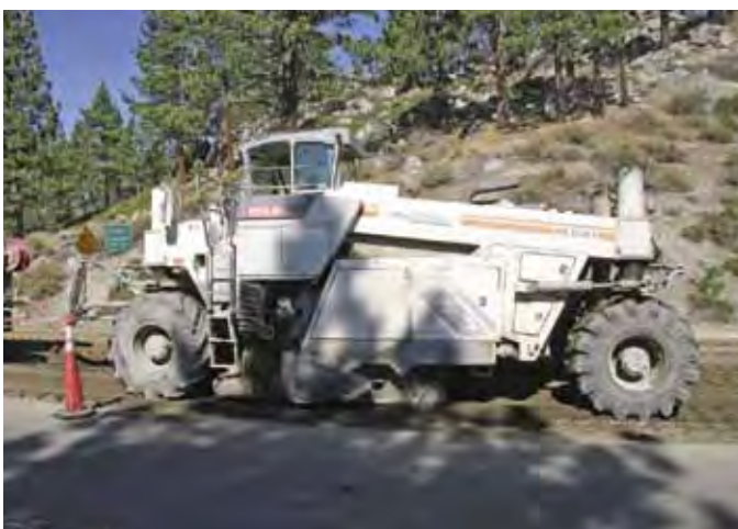
Pulverizer Operator Nick Warren mixes concrete with base as he rolls down the highway.
