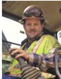
Chris "Butch" Biagi performs clearing and grubbing for Tyrrell Resources, Inc. on the Lance Gulch Road project.
