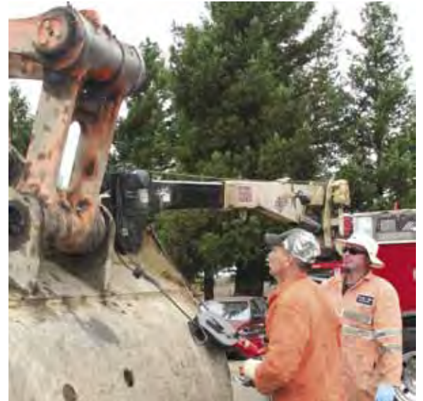
From left: Mechanics James Noah and Greg Driscoll put together an excavator on the giant subdivision job for DeSilva Gates in Rohnert Park.
