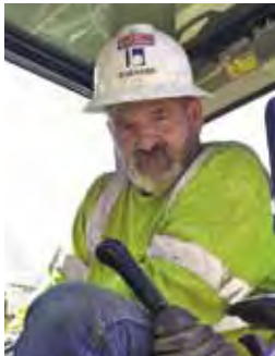
Rodney Taylor works for Tyrrell Resources, Inc. in Weaverville, clearing the jobsite on the Lance Gulch Road project.
