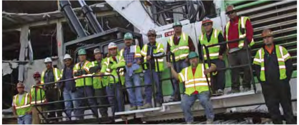
Operators Rich Capaldi, Jim Wagner, Fred Wolovic, Tim Pasley, Alfredo Pena, Manuel Rodriguez, Jose V. Cisneros, Jose G. Cisneros, Jose Cisneros, Victor Gomez, Ben Villasenor and Jose Perez and apprentices DagoBerto Uriarte and Adam Jacobs work on the demolition of the Downtown Plaza for Ferma Corp.
