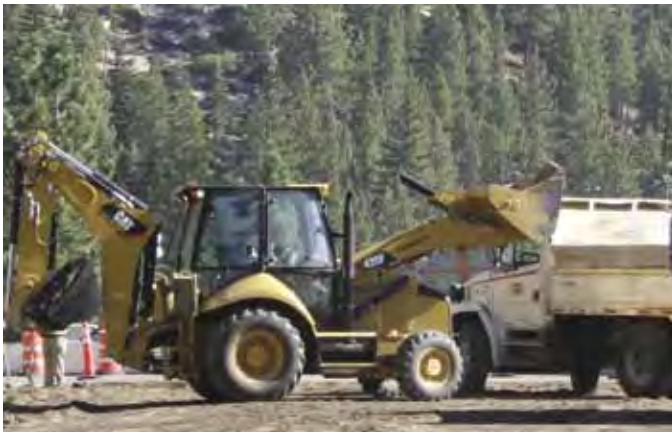
Rubber Tire Backhoe Operator Bill Rushford picks up asphalt chunks, so the Concrete Treated Base (CTB) can be laid.
