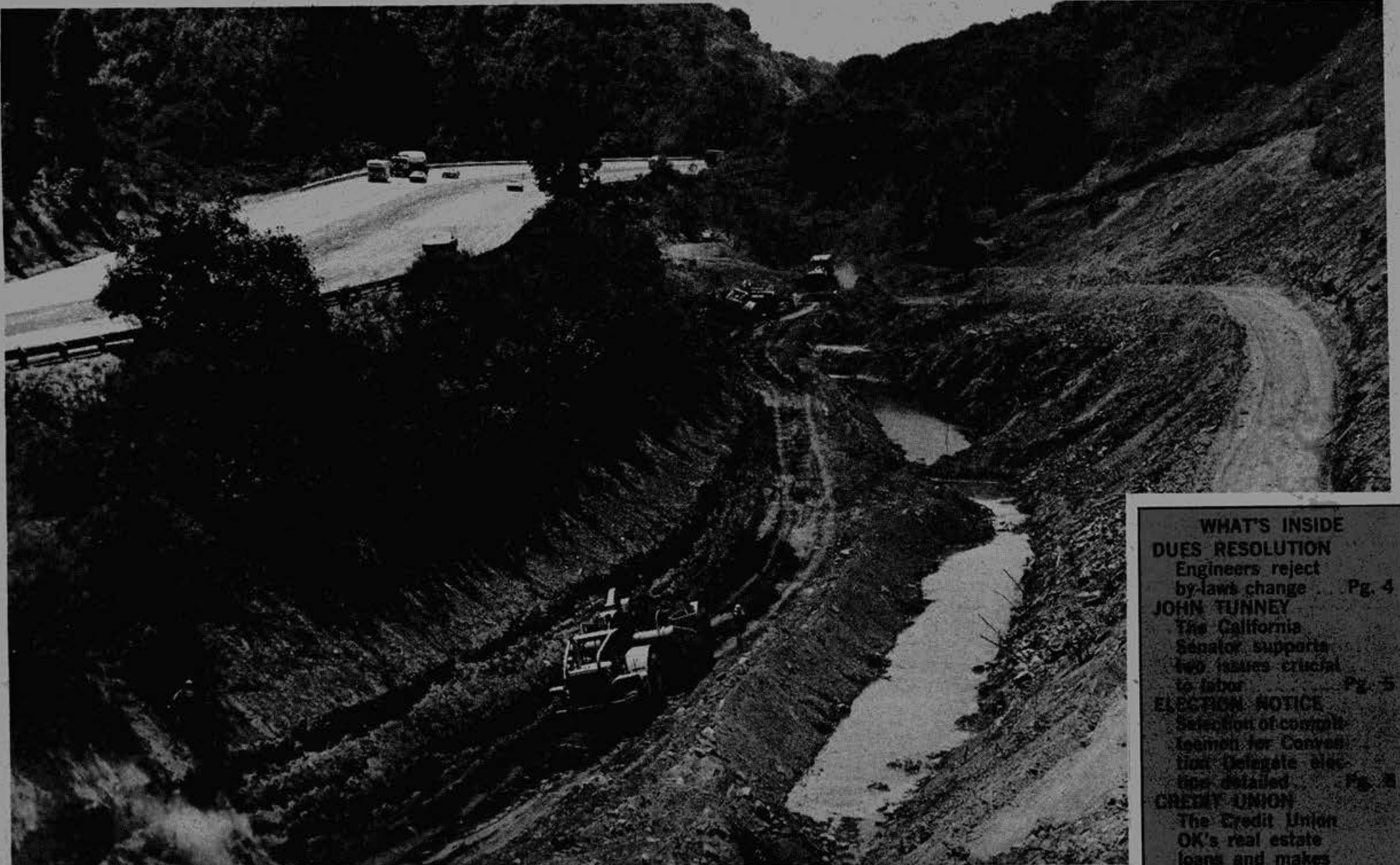
OPERATING ENGINEERS at work on the first of three phases of the $90 million I-580 job in Alameda County.
