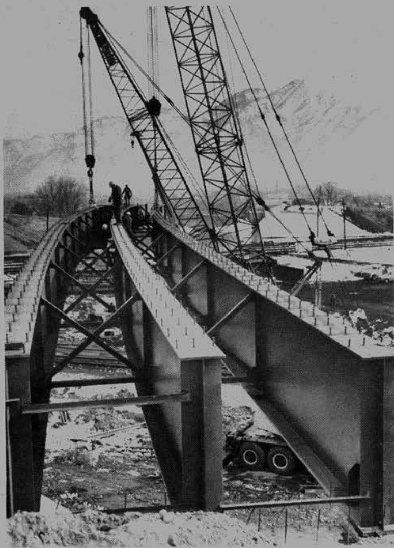
THE FOUNDATION FOR the eastbound lane of the 20th-21st Street Project in Ogden, Utah is taking place as steel girders, 7½ feet high, are put in place. Total cost of the project is $6.5 million.
