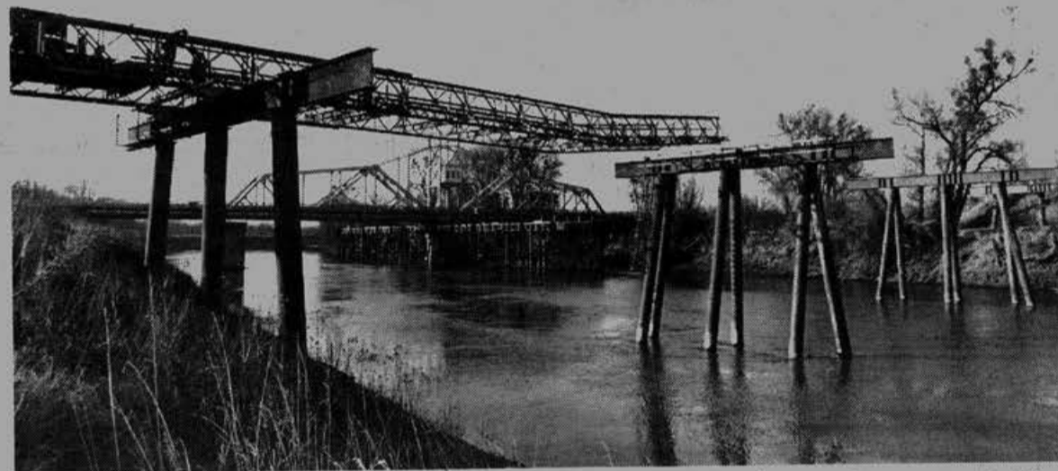
THE END IS NEAR for the 64 year old Meridian Bridge over the Sacramento River on
