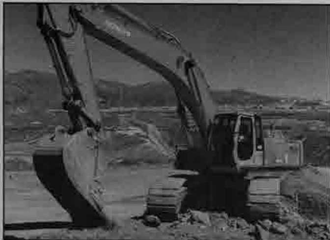
SCENIC SETTING: Against the snow-capped Sierra Nevada, Operating Engineers put equipment through the paces.
