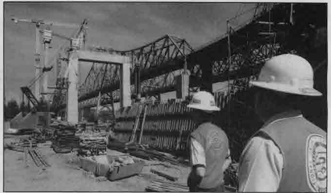
Fairfield Assistant District Rep. Bran Eubanks and Organizer Justin Diston assess progress at the Carquinez Bridge.
