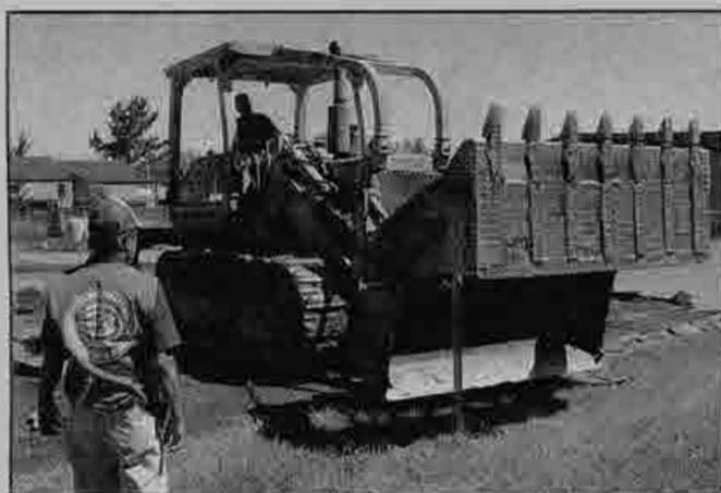
▲ Retiree Leon Calkin, who did some of the gradesetting for the project, directs loader operator Tom Wilson of North Bay Construction.
