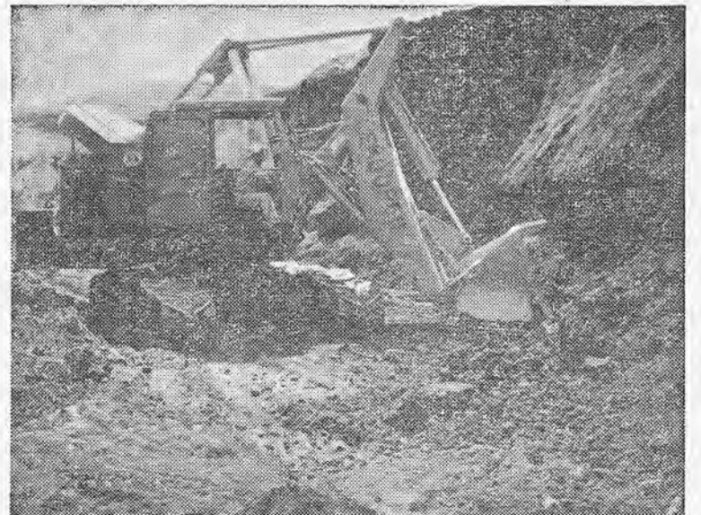
NEW EQUIPMENT —Koehring Scoopers are included in new equipment on the Green, Winston Camanche Dam job. The machine is a yard and one quarter Koehring, with a four-yard loader front, hydraulically controlled. More than $2 worth of equipment is involved in the Camanche project.
