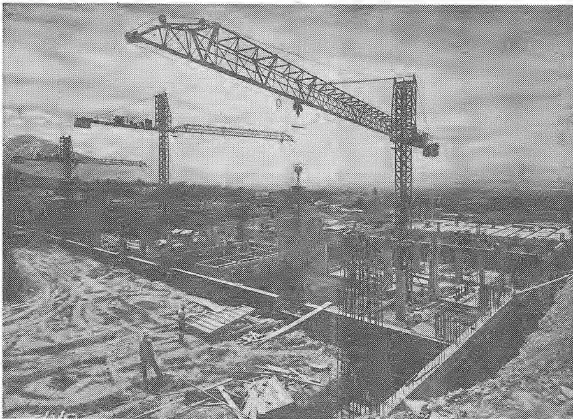
THREE OF A KIND —Three Linden cranes are being used on the Medical Building on the University of Utah campus. Prime contractor on the $6½ million project is Christiansen and Paulsen. Building will have five stories above ground. Center crane boom is about 10 feet higher than others. Leroy Mitchell is operator of the center crane, with Roland Johnson and Sven Ronning on the other two. They're keeping up with rapid pouring schedule.
