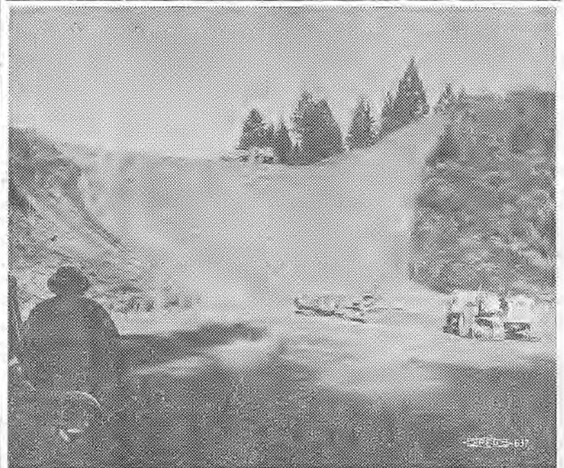
SLICING THRU SIERRAS—Up where the timber line starts, around Colfax, the construction industry is taking first big steps toward lightening the impossible traffic burden on mainline Highway 40, the road to Reno. The goal is doubletrack all the way over, and the Federal Highway Program will no doubt speed up this goal, especially prior to the 1960 Winter Olympics at Squaw Valley. McCammon & Wunderlich have a 6-mile, $3,601,981 contract at Colfax.
