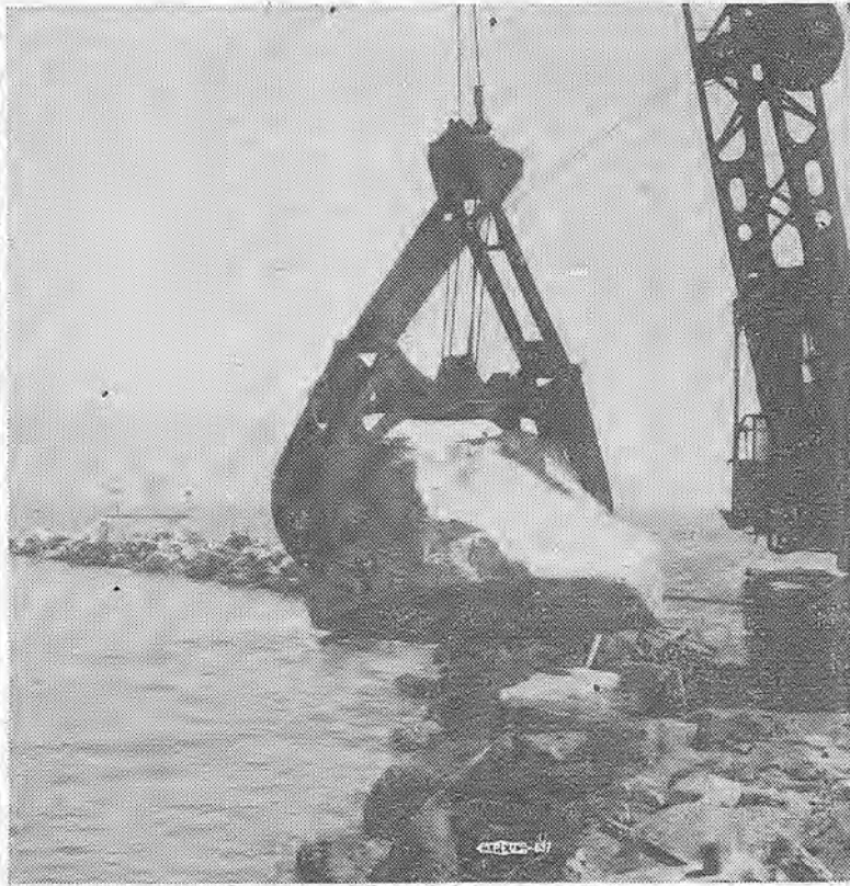
UNIFORM STRAIGHT-TIME rates would be in effect throughout the area, on a yardage basis, for shovels, cranes, drag lines and clam shells under the Local No. 3 proposals. Lower rates for counties outside the Bay Area would be upgraded.
