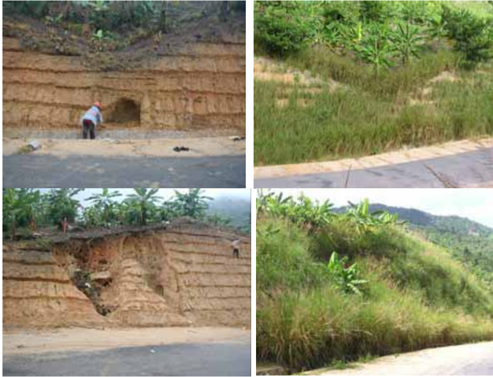
Photo 22: Pham Hong Duc Phuoc, a road protection project in Khanh Hoa province, road to Hon Ba): left two Photos: severe erosion on newly built batter occurs after only a few rains; right two Photos: eight months after Vetiver planting: Vetiver stabilized this slope, totally stopping and preventing further erosion during the next wet season
