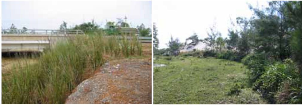
Photo 6: Left: Vetiver protects bridge abutment along Nat. Highway nr.1; right: December 2004, local species have replaced Vetiver
