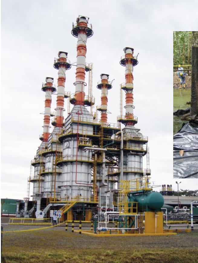
The OCP facilities at Lago Agrio.
