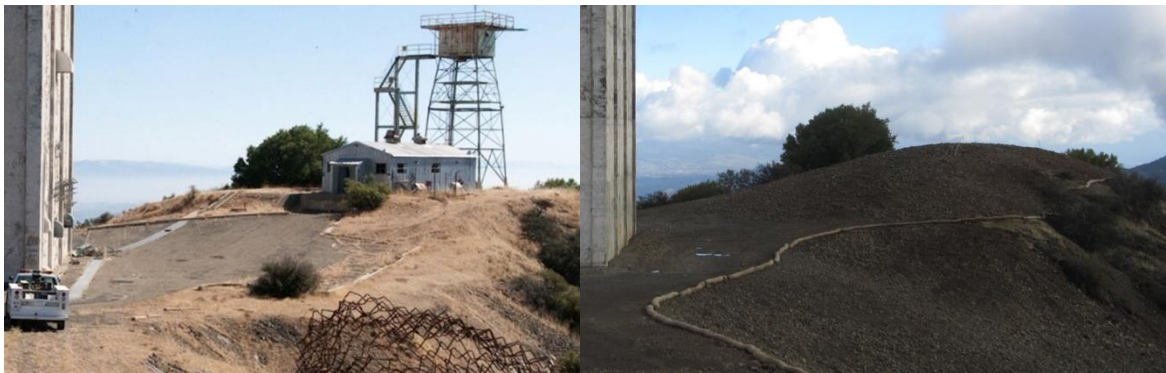
Figure 5: Before and after photos of re-contoured east summit area after rough grading and structure removal. Grading will be refined in 2016-2017.
