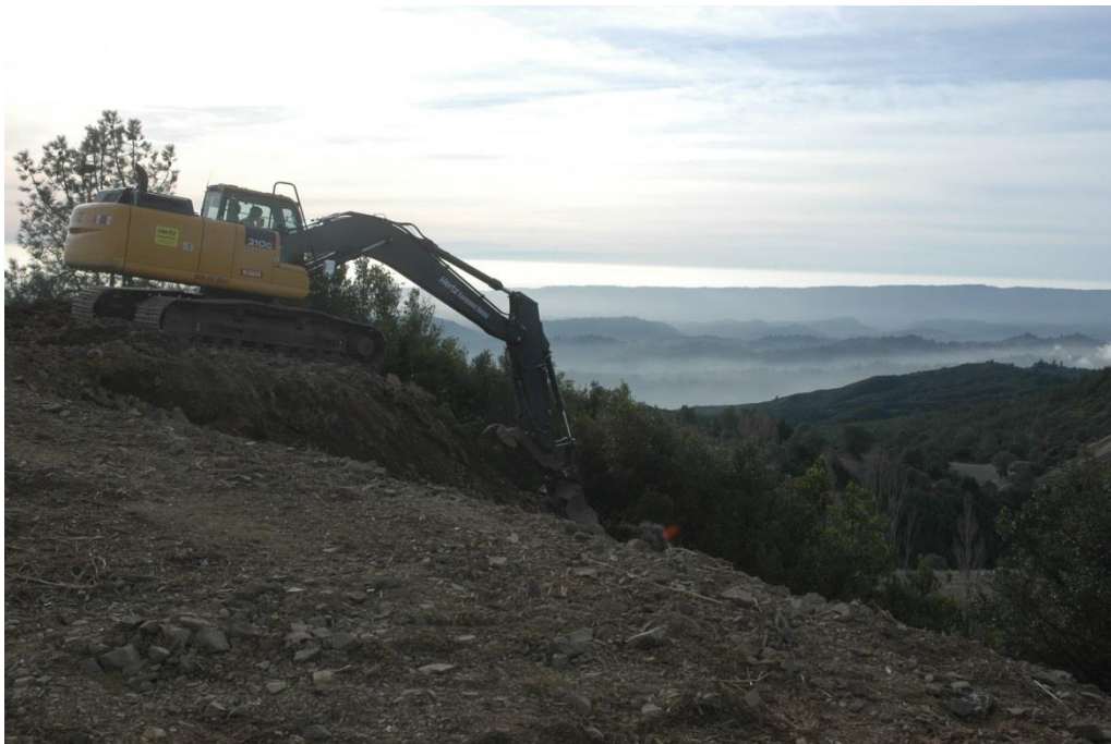
Figure 2. As the vegetated edge of the summit is pulled back, the existing root channels and soil structure is mixed. Existing root channels and drainage pores are destroyed. Mixing of coarse wood materials and care to not re-compact the substrates are the primary treatments to regenerate pore space for root growth and drainage.
