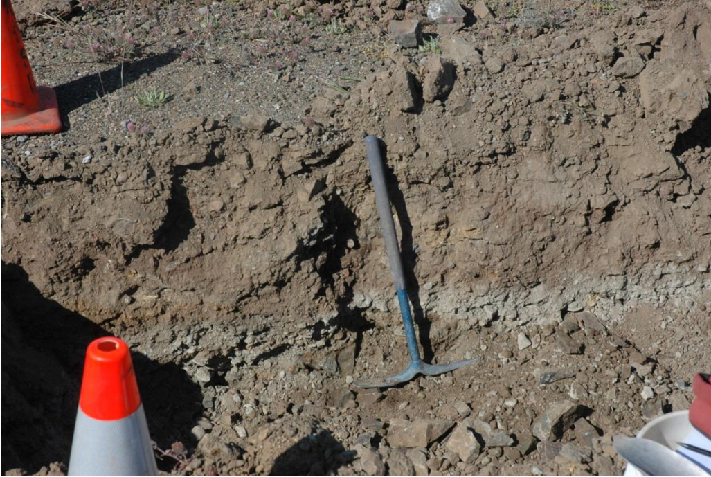
Figure 3. Existing or regraded areas of excavated soils have various dense subsoil layers or are compacted. A final re-excavation, mixing of coarse organics, and replacement without compaction are basic treatments to regenerate infiltration and allow root growth to re-enter these substrate volumes.
