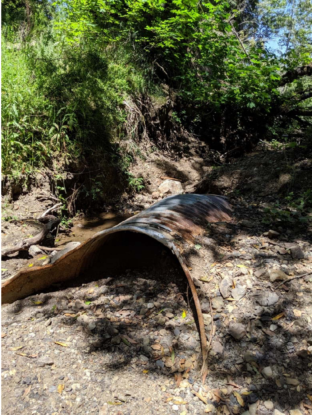
Photo 3. Delineated other Waters at Data Point P01, looking west to east across study area corridor, showing damaged, non-functional culvert in stream channel.
