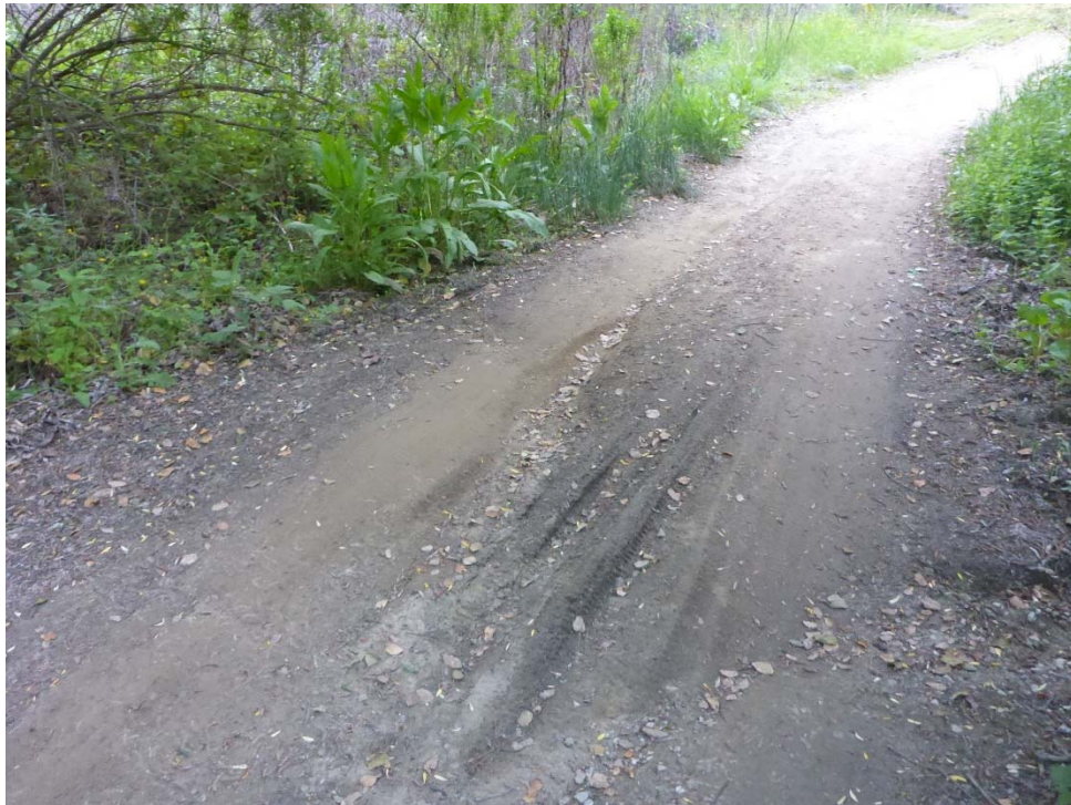
Photo 6. Representative photograph of access road within study area, showing minor rills from sheet flow after heavy rains.
