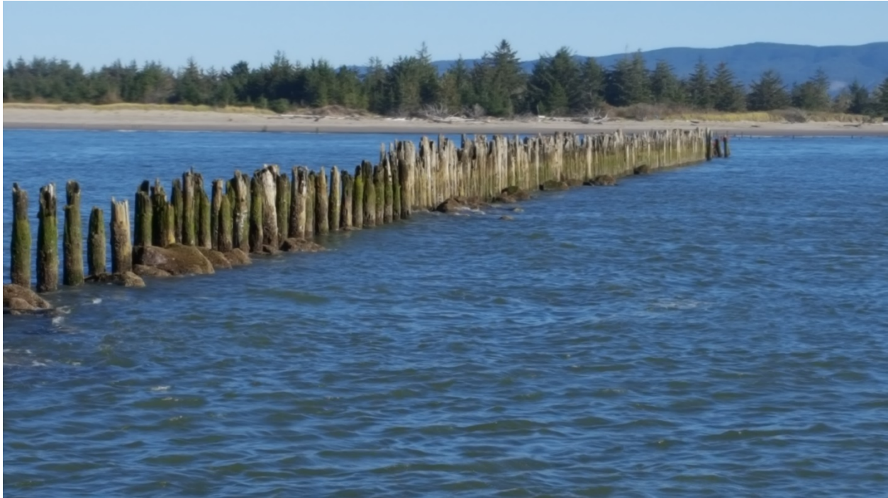
Figure 2. Deteriorated Condition of Baker Bay Pile Dike (October 2017)
