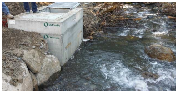
The new concrete vault diversion structure provides water through screened openings below the waters surface.
