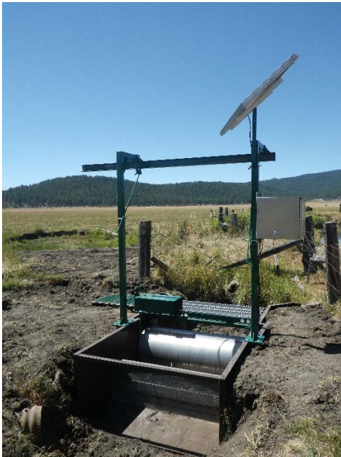
A solar system provides power to a screen where low flows make use of other power options inadvisable.
