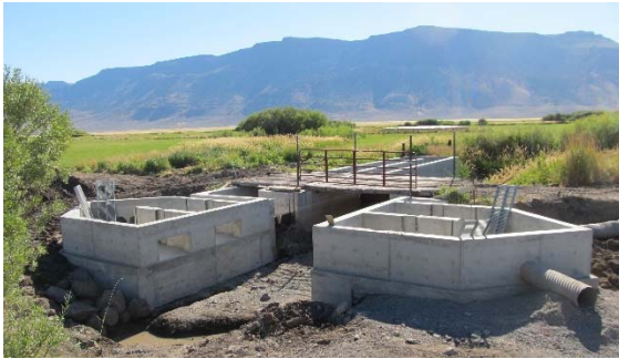
Taken during construction, this photo shows both diversion structures. Honey Creek will flow between the concrete structures.
