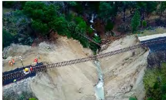
Union Pacific used drones to assess weather-related damage in Doyle, California.
