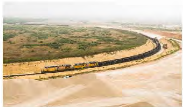
Building a 12-mile stretch of Interstate 69 in Texas recently required more than half a million tons of Martin Marietta's aggregate moved on Union Pacific trains.
