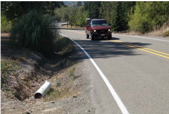
No shoulder and drainage ditch along Tiller Trail Hwy north of Strongs Market.
