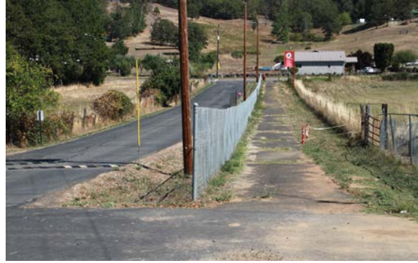
Sidepath adjacent to school driveway is overgrown with weeds and cracked pavement.
