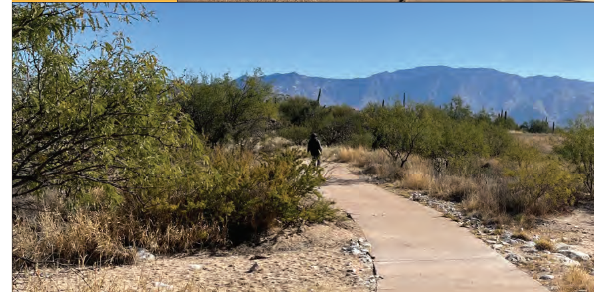
EXISTING CART PATH CRACKING
