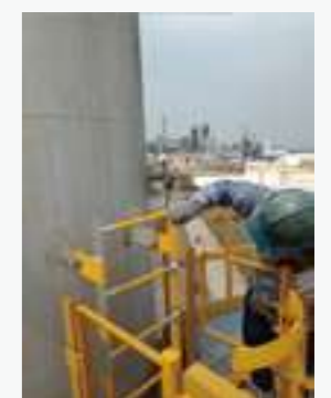
The platform ladder is added with a crossbar extending at least 60 cm above the platform
