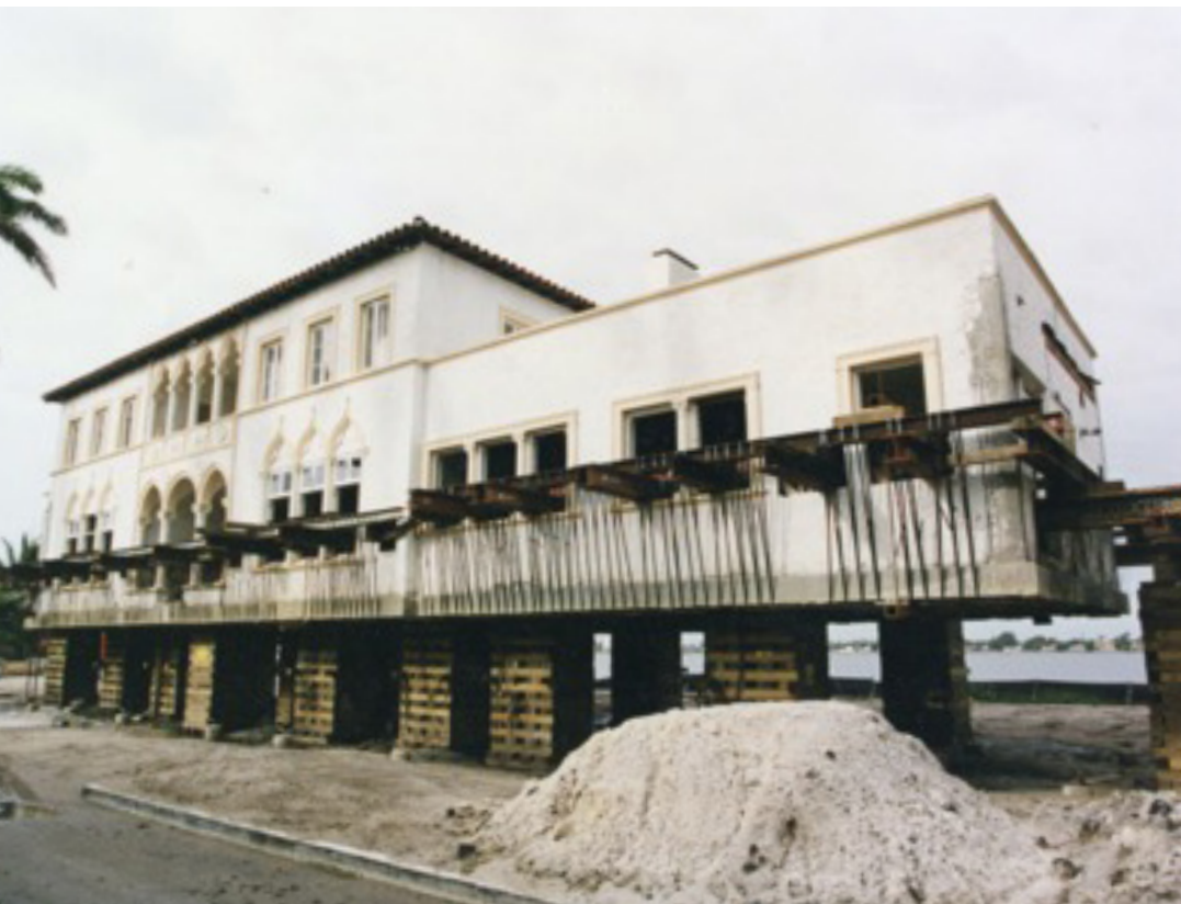
Villa Tramento on Clarendon Avenue being raised to prevent further flooding damage. Image by Gene Pandula.
