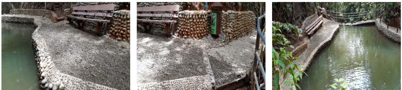
Figure 6: Rock lining on both sides of the 1st pool and also on the walkway and side walls.
