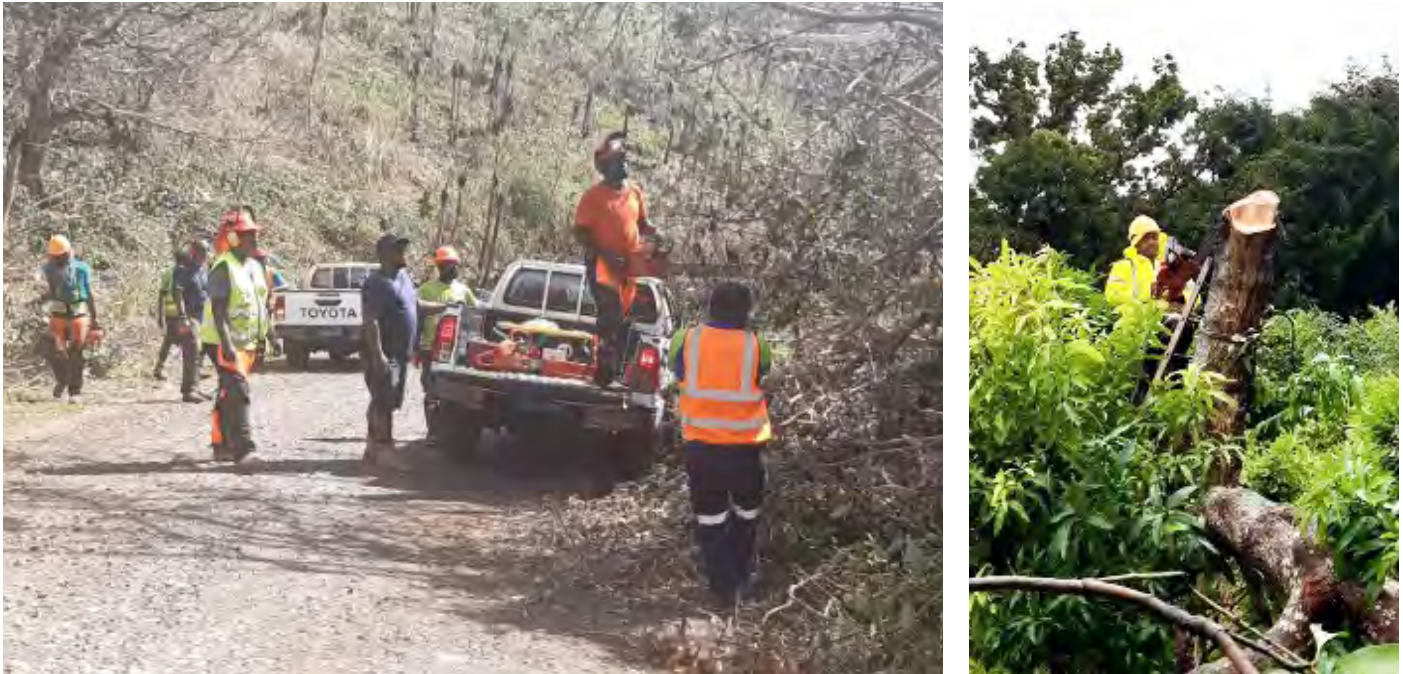
Figure 21: Staff clearing debris and fallen trees after cyclones
