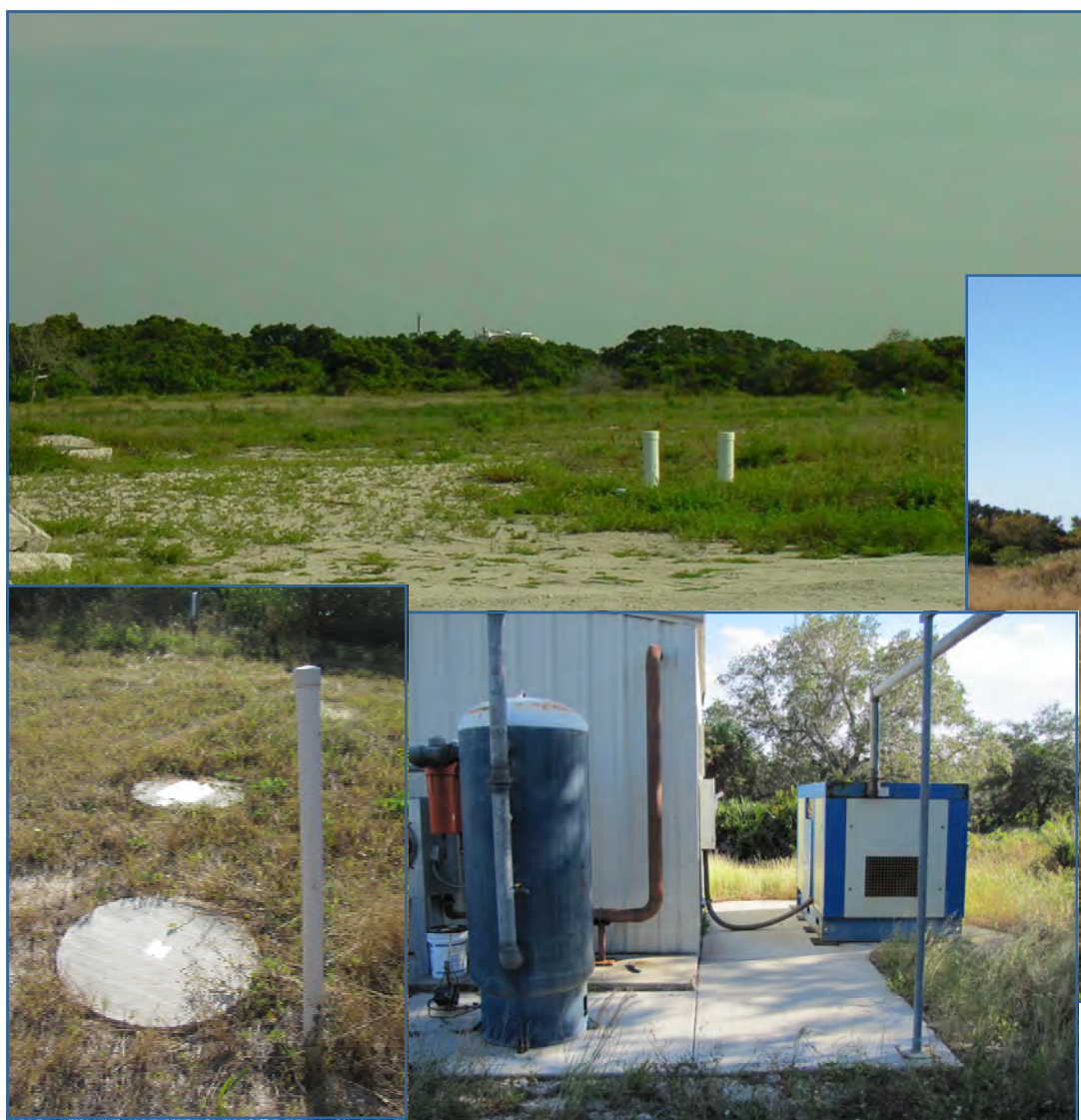
Left: The grassy area in this photo was cleaned up as part of the solvent extraction Interim Measure. This photo was taken from the road leading into FT017 facing north, shortly after the cleanup.
