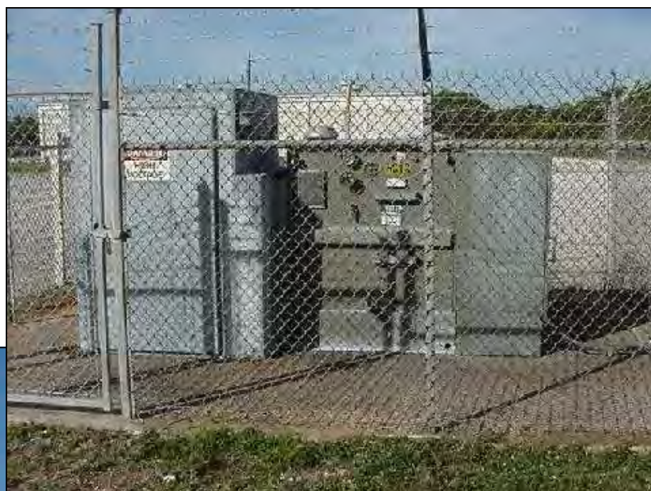
At left: Transformer Substation, Facility 7802, where Hangar C assessment originated. Transformer is located on southwest corner of Hangar. Groundwater contamination is also on that side of the hangar.
