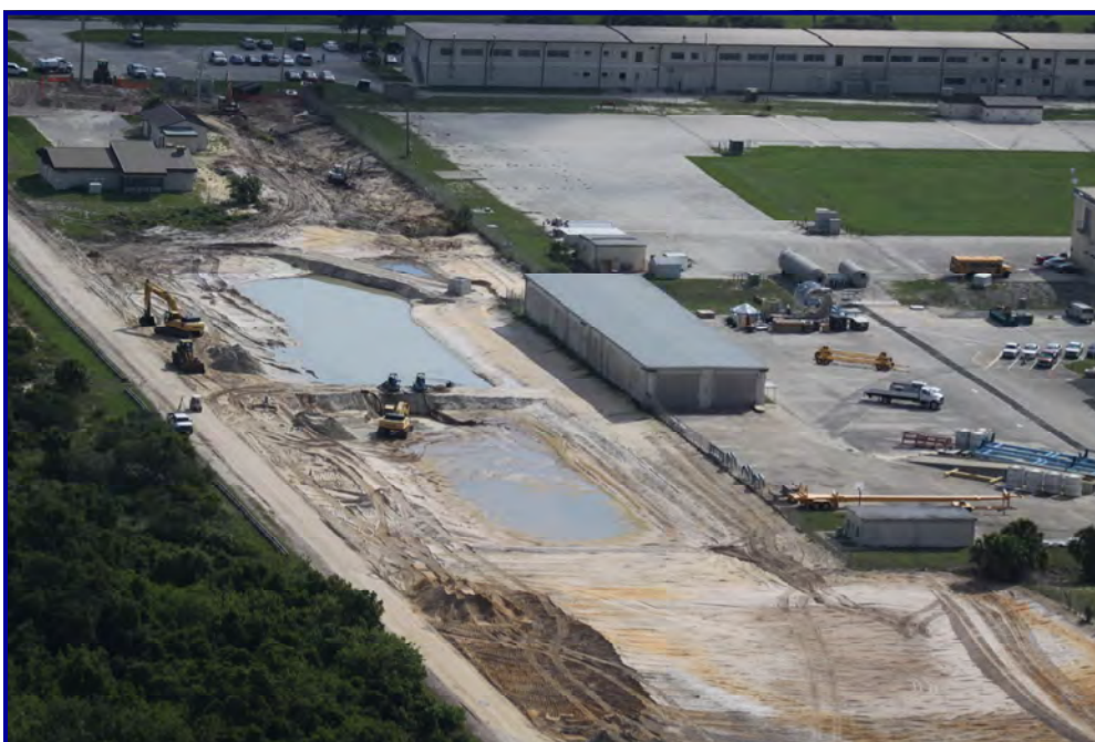
Upper left: Construction of primary treatment basin—a pond of approximately 12 acres, located just west of CCAFS Industrial Area (approx 2010).
