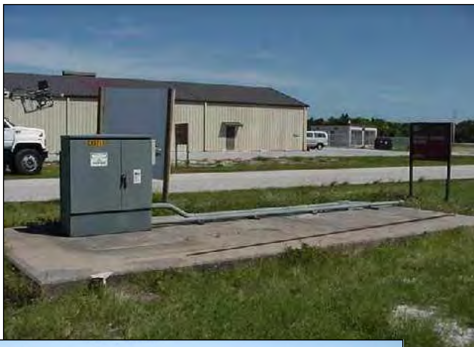
At left: Close-up of transformer where the Facility 38320 Area investigation started. (Photographer was standing in front of Facility 43400, looking southwest across Beach Road.)
