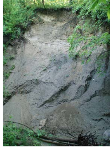
Bank failure on creek
