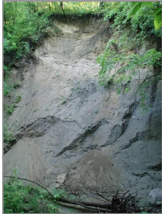
Figure 37 Site 11 noted slope failure immediately adjacent to the stream
