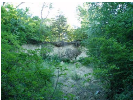
Large slope failure has wet soils on lower area, very dense sandy clay soils on upper bank.
