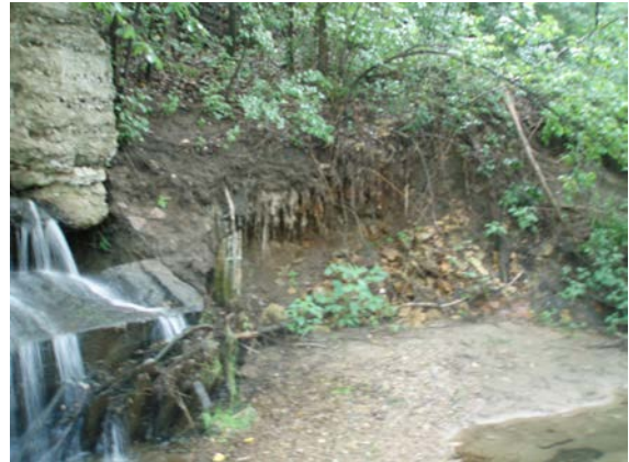
Large bank failure downstream of culvert outlet on left bank
