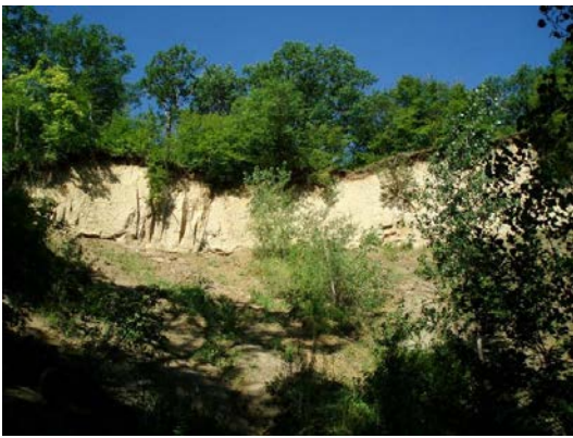
Large slope failure has wet soils on lower area, very dense sandy clay soils on upper bank.
