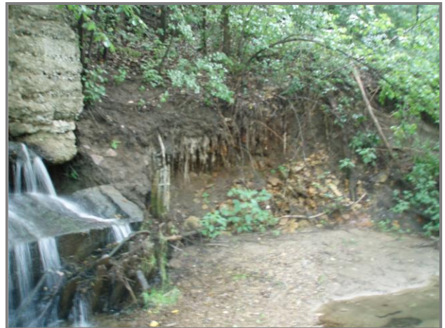
Figure 35 Streambank erosion is undermining this culvert at Site 1.
