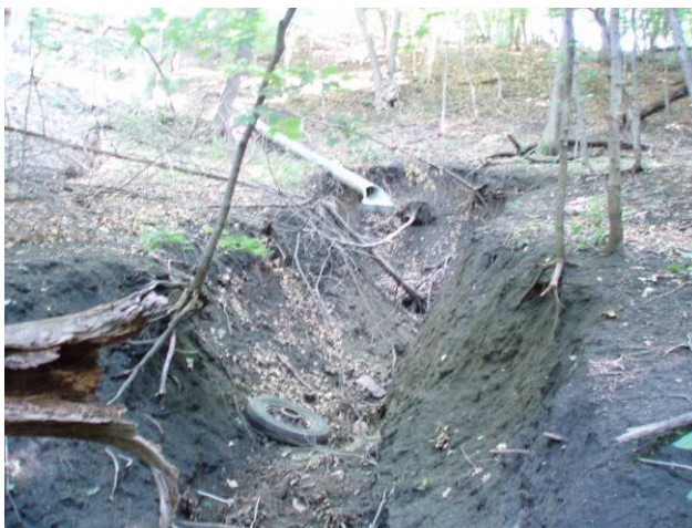
Large headcut in main ravine below pipe outlet from Mandan Circle
