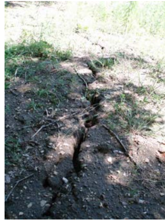
Crack foretells impending slope failure
