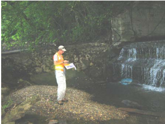
Large drop and undermining at downstream end of regional trail culvert
