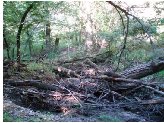
Timber debris and sand deposit at channel bend
