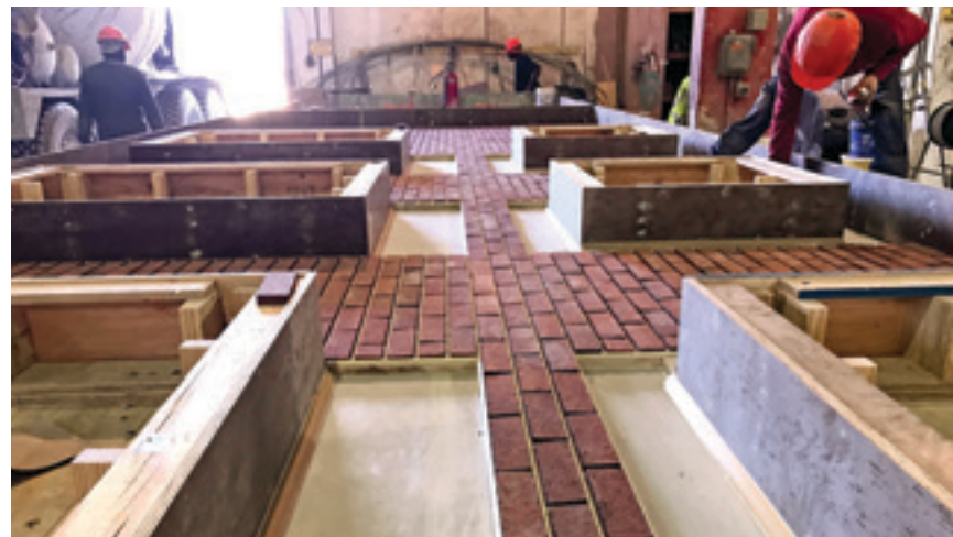
Thin bricks are assembled in the bottom of the form, ready for the precast concrete to be placed. Photo: Coreslab Structures (Indianapolis).
