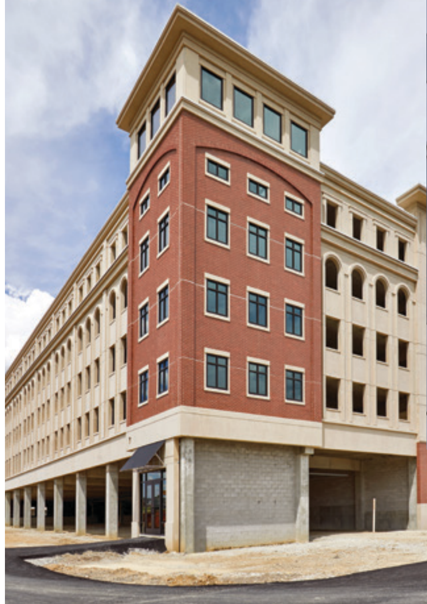
Precast concrete panels on the cast-in-place frame helped meet the aggressive schedule. Erected in just seven weeks, the precast concrete installation took place during the winter of 2017, with the entire parking structure constructed in one year. Photo: Tony Frederick Photography.
