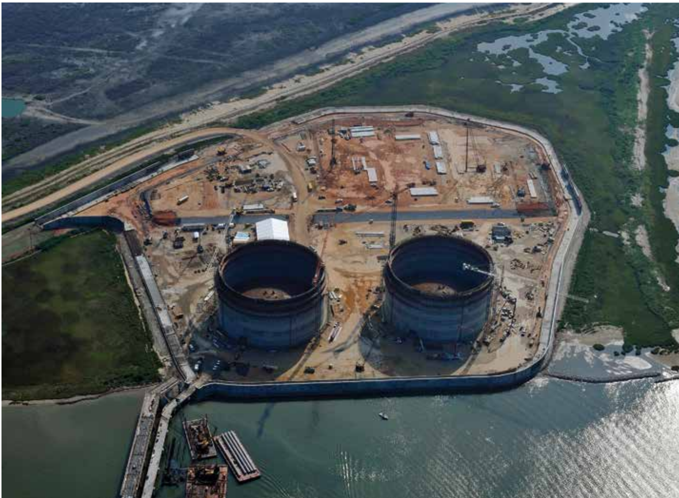
Figure 1. A typical liquefied natural gas (LNG) receiving terminal showing the marine berths for the LNG carriers and the LNG storage tanks and associated regasification equipment under construction. The secondary containment roof has not yet been constructed.
