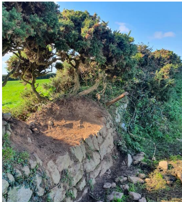
Erosion of a Cornish hedge with furze hedgerow at Raginnis, Paul illustrates its construction with battered, roughly coursed stone faces and tamped rab core.
