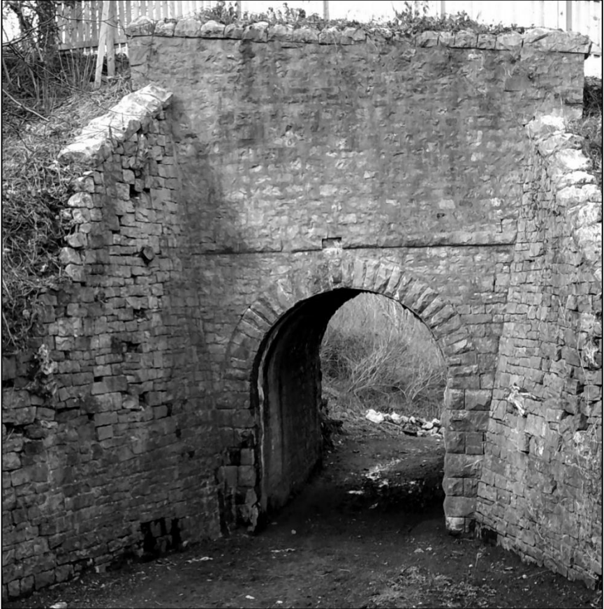
The reverse side of the Gethin Colliery tramway bridge that carried coal between No.1 & No.2 Gethin pits. Photographed 05/04/2018.
