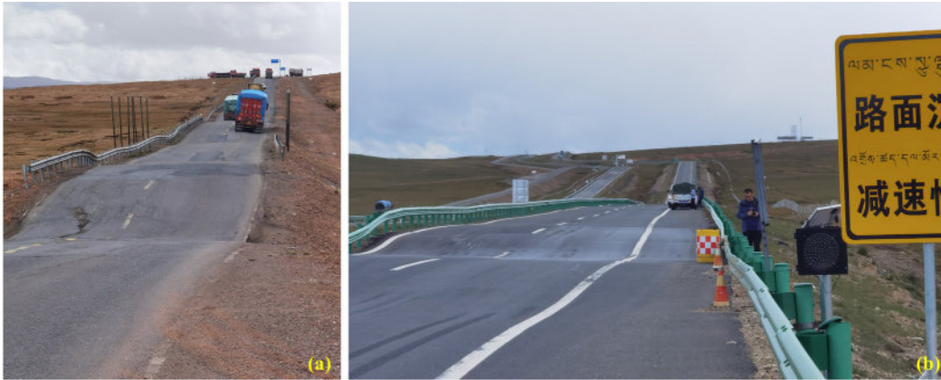
Fig. 15. Thaw settlement in the highway embankments in permafrost regions of the QTP. (a) Serious thaw settlement in the old Qinghai-Tibet Highway embankment; (b) Thaw settlement in the new constructed GYE.
