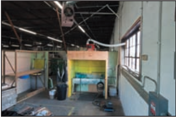
This silkscreen cleaning station, situated at the rear of the building to reduce noise levels, is 100 feet from the nearest drainline. Rather than break up the floor, Kolbi installed a Sanicubic system that pumps wastewater 18 feet up to a horizontal main at the ceiling.
