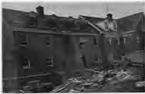
Construction progresses on the addition to the Phi Psi house at West Virginia University.
