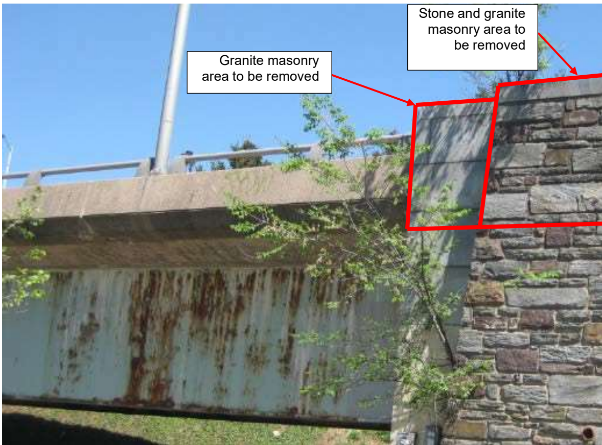
Photo 2 - Existing Girder, Outside Barrier, and Wingwall. Areas of abutment and wingwall to be removed will be replaced with concrete barrier. The inside and outside faces of concrete barrier will be faced with salvaged stone. New stone that is similar material, color, size, and shape will be used as needed.
