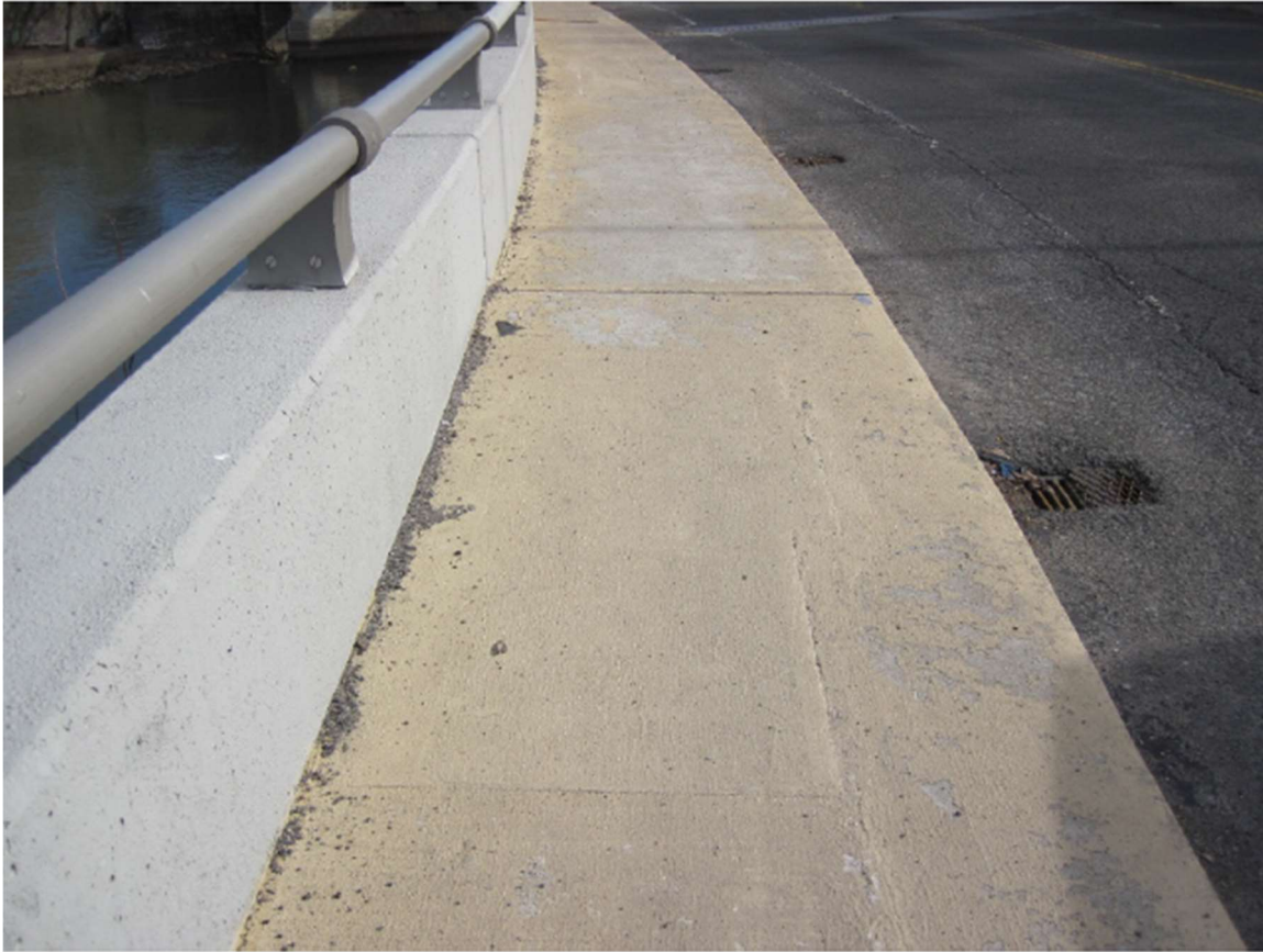
Photo 5 - Existing Sidewalk on Upstream Side and Inside Face of Barrier
