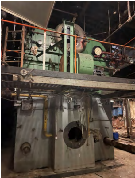
Figure 9: Existing boiler compromised by Hurricane Ida.
