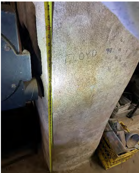
Figure 5: Highwater mark within the building for Hurricane Floyd (1999).
