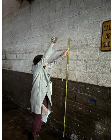
Figure 3: Highwater mark within the building for Hurricane Ida (2021).
